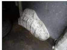
Door R R, Damaged, LI - Repair and paint (complete) 238,76
