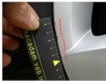
Roof, Dent(s) and scratch(es), LI - Repair and paint (complete) 481,50
