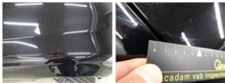
Ceiling, Hole, Smart repair
