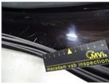
Roof, Chemical pollution, LI - Repair and paint (complete)
