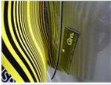
Floor covering F L, Hole, E - Replace
