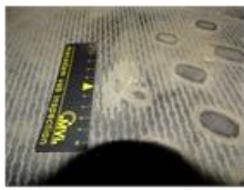
Wheel cover R R, Broken, E - Replace
