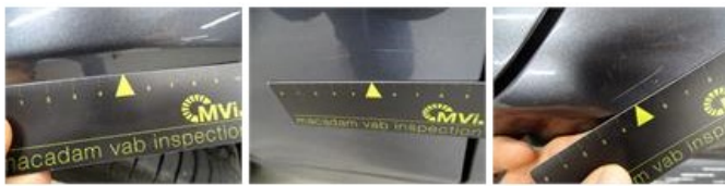
Roof, Chemical pollution, LI - Repair and paint (complete)
