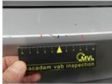
Ceiling, Stain, Cleaning
