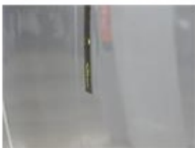
Roof, Chemical pollution, LI - Repair and paint (complete)
